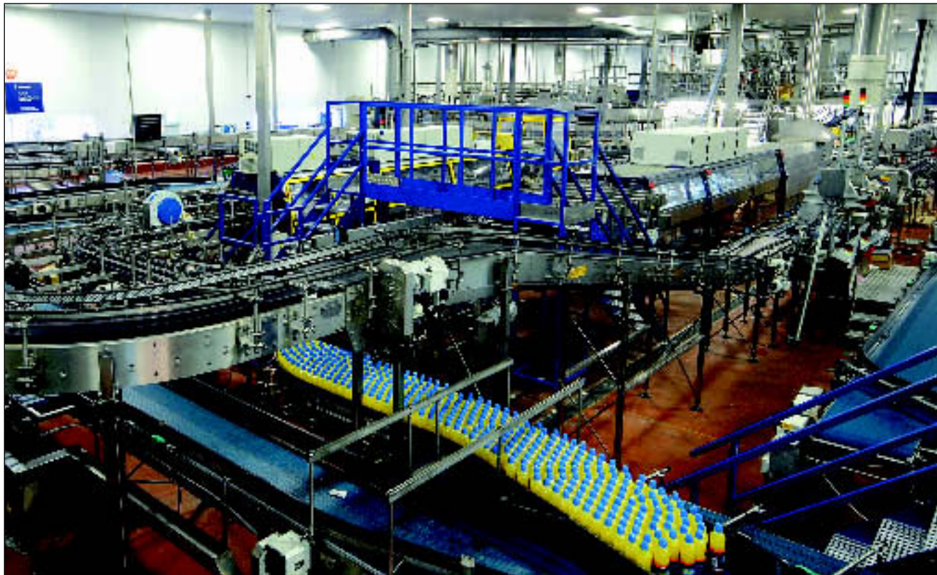
The packaging hall at GlaxoSmithKline's plant includes sleeving equipment from Fuji Seal and shrink wrappers from SMI
